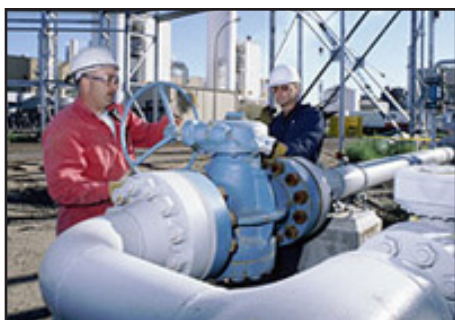
Weyburn CO 2 project. (photo: NETL)
